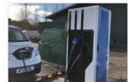
DC EV chargers
